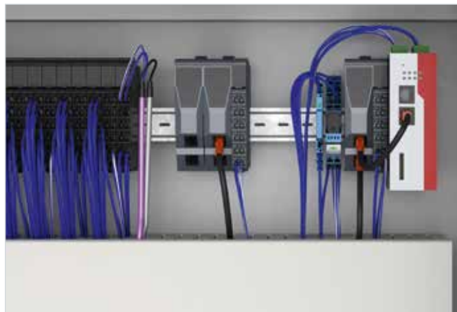
VPN router for remote maintenance (remote collaboration)
